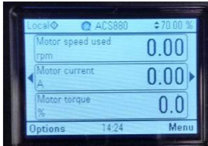
Figure 15: VFD Interface in Local Mode
